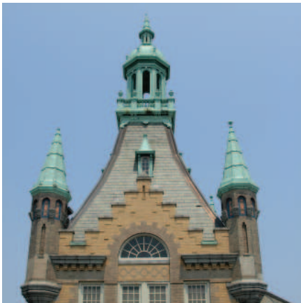
Top, left: Tower before restoration. Top, right: Tower after restoration. Bottom: Turret roof after restoration.
